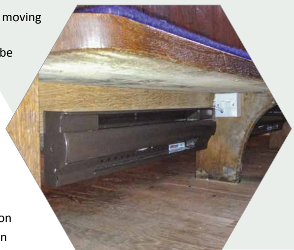
SKL heaters installed under pews
